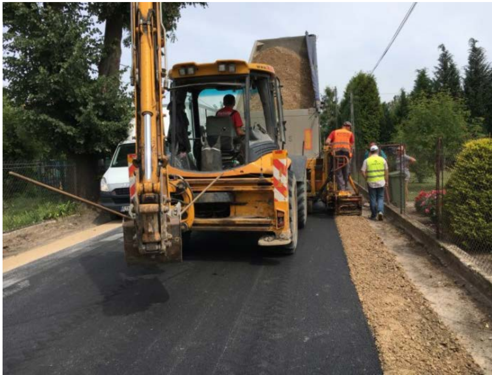
Figure 2: Construction of trial road in Poland where bio-based lignin has been in the asphalt. (Source: https://apseproject.eu/5704 )
